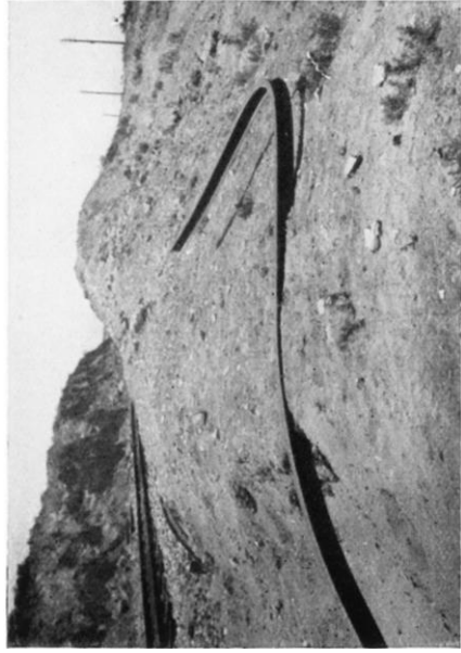
3. Twisted rail near Mastung W. D. W.
